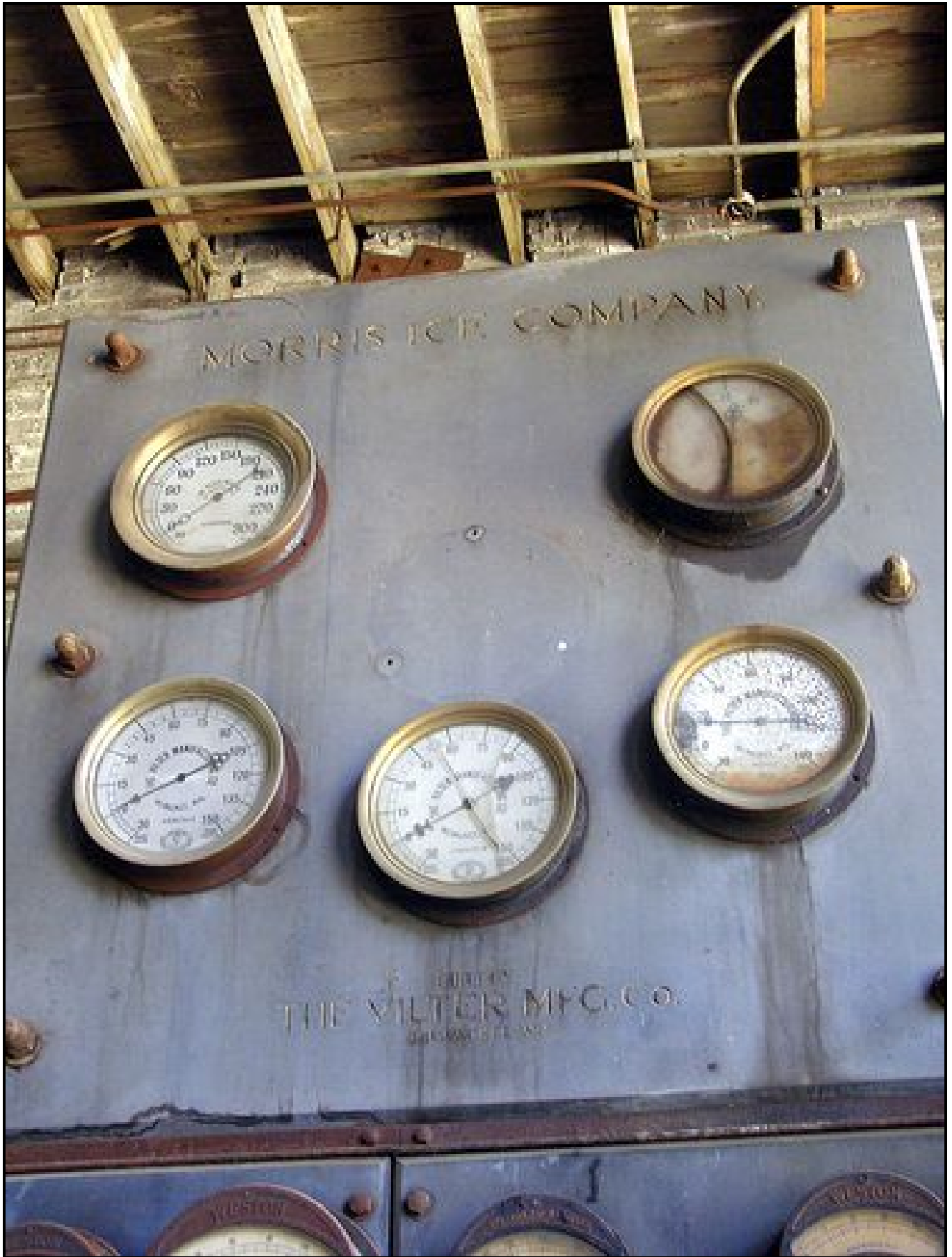
Vilter Refrigeration gauge board at Morris Ice Company
